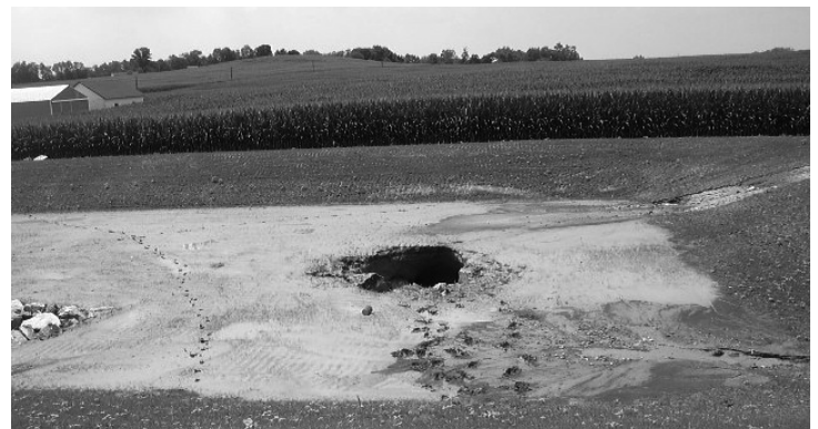
This small sinkhole appeared in a stormwater detention basin.
